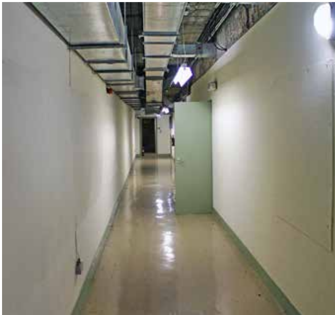
View of upper corridor showing ceiling mounted ventilation ducts and exposed in-situ concrete roof at high level
